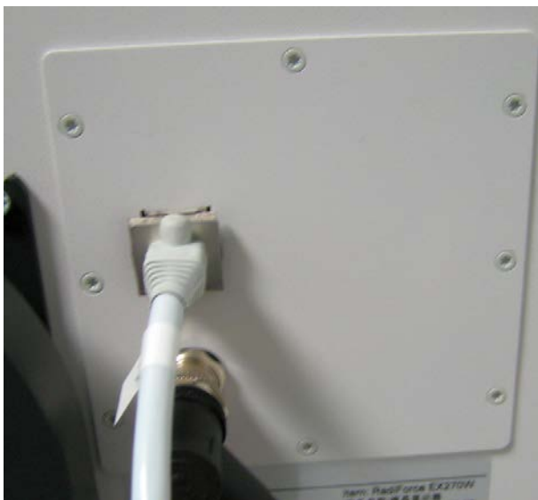
Fig.: Installed EMC pad and holding plate on the TRM0000-TDL input module
